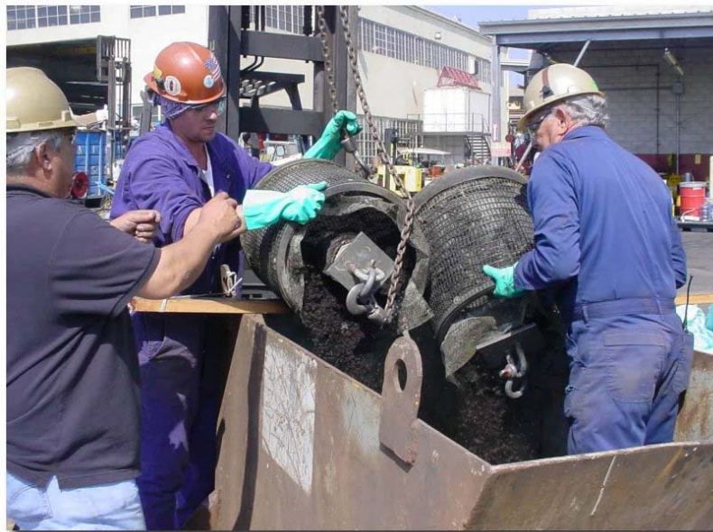
Maintenance personnel changing the SWFS filter media.
