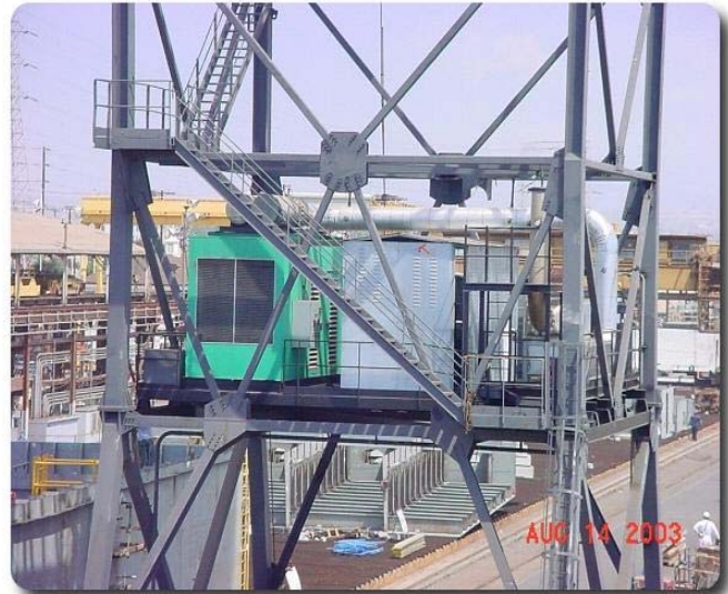
Crane # 12 with the new engine (in the left enclosure) and the air pollution control equipment on the platform.
