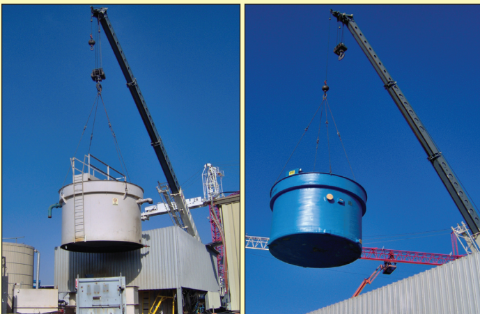
The removal of the old Dissolved Air Flotation Tank (left) and the installation of the new composite tank (right).
