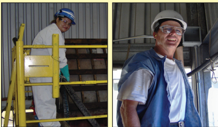
Juanita Espinoza cleans the oil/water separator (left) while electrician Jorge Barragan replaces electric lines.
