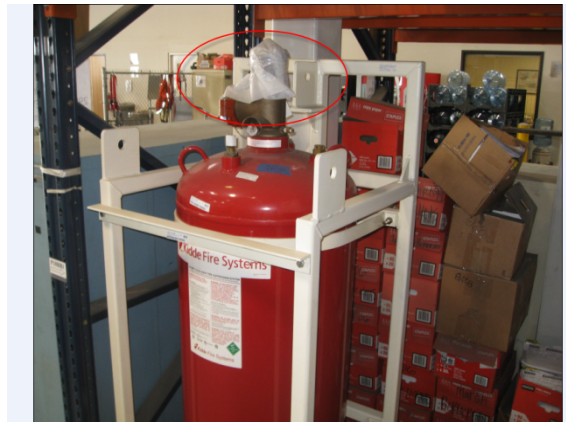
See above for a correct example of proper protection for a coupling or gauge.
